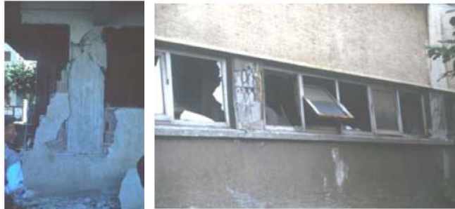
Figure 3: Columns shear failure during earthquakes
