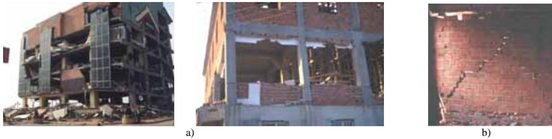
Figure 1 – Damage on masonry infill walls (Varum, 2003): a) RC frame building with almost fully damaged masonry infills; b) diagonal tension failure of a masonry wall
