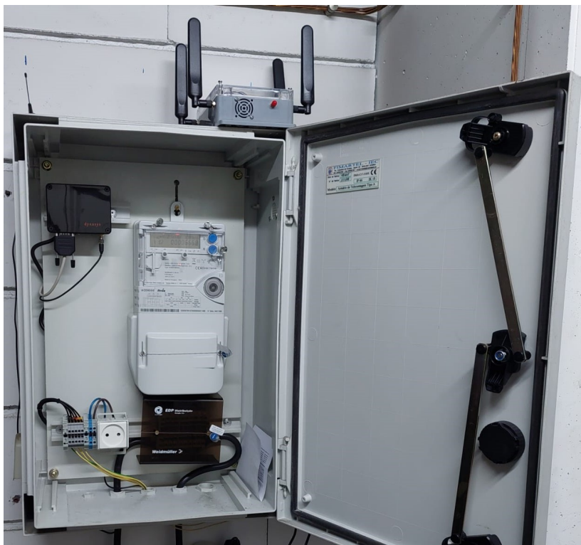
Figure 4.3: Smart meter installed in a medium voltage system.
