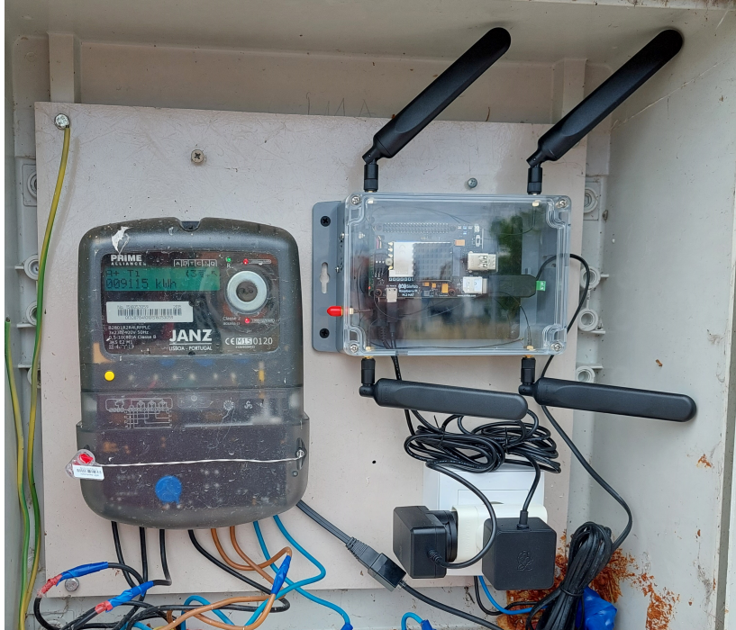
Figure 4.2: Smart meter installed in a low voltage system.
