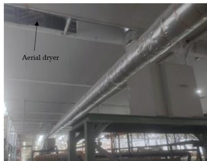
Figure 12. Conducts in link from the oven continuous to the air dryer.
