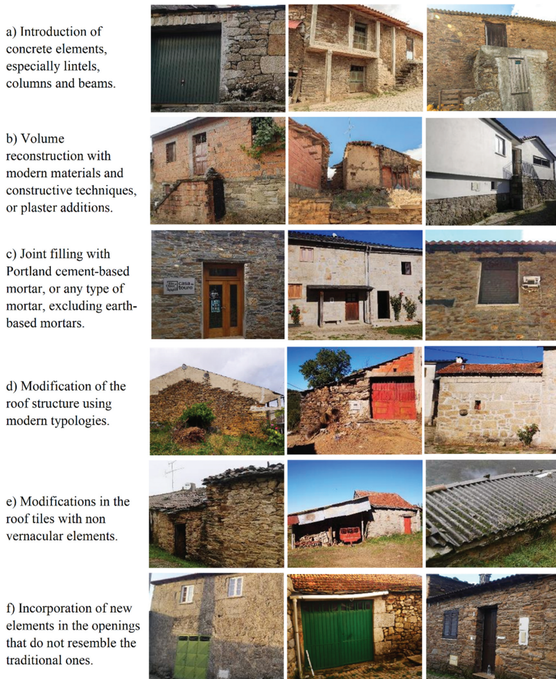
Figure 5. Examples of the main “dissonances” found in Montesindeho Natural Park buildings.
