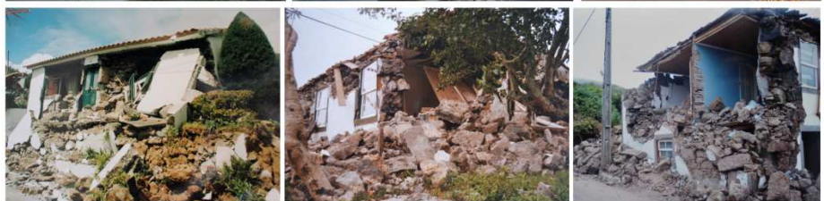
Figure 5. Examples of evaluated buildings belonging to each damage grade from the EMS-98 scale
