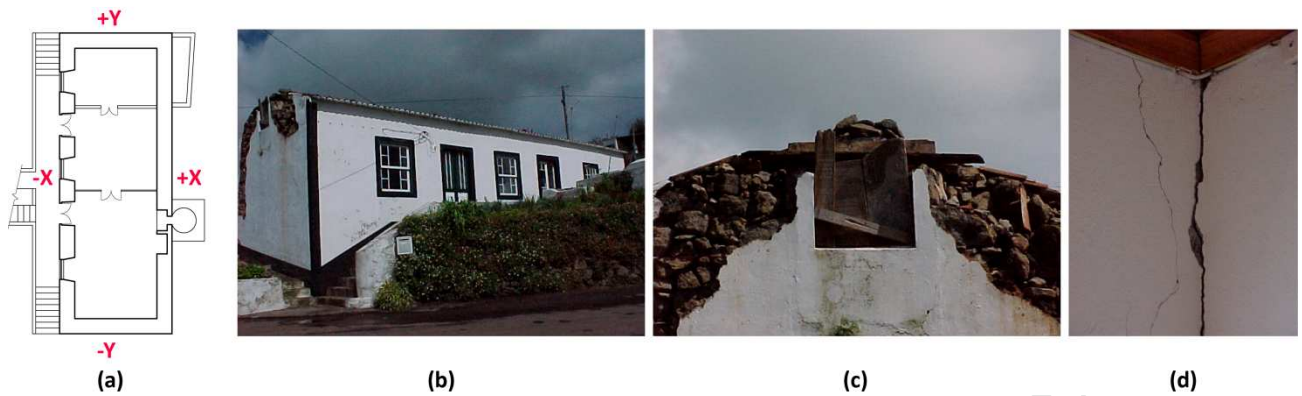
Figure 18. (a) Building plan and directions nomenclature; (b) main façade of the building; (c) collapsed gable wall; and (d) visible damage at the wall-to-wall connections from the interior of the building
