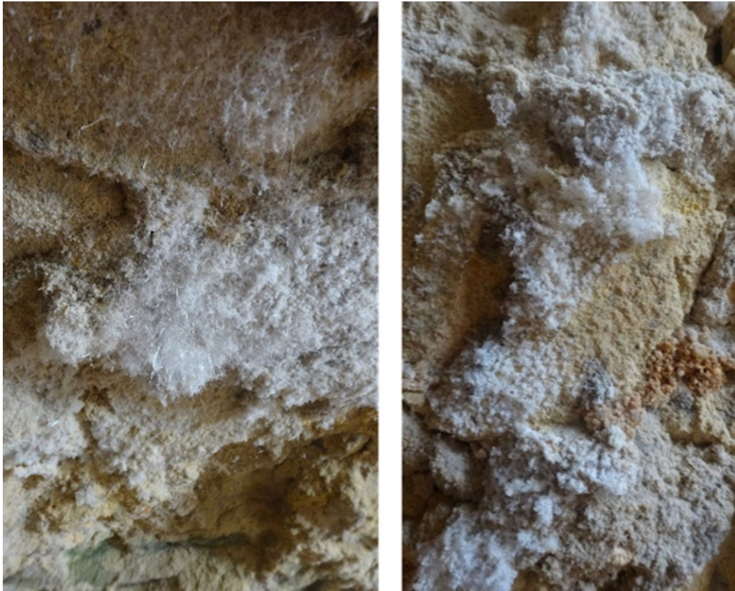
Fig. 10. Presence of efflorescent salts in different locations on the formed wall, image height match: left - 6 cm; right - 36 cm (© Alice Tavares).
