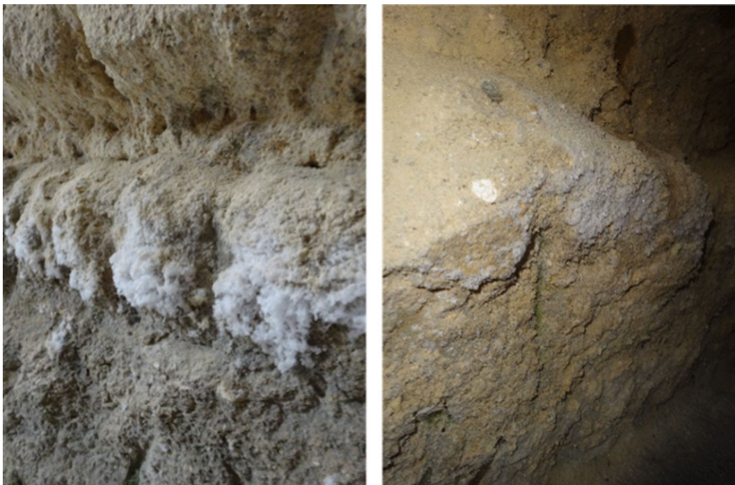
Fig. 11. Presence of efflorescent salts in different locations of the same row of the adobe wall, image height match: left - 45 cm; right - 50 cm (© Alice Tavares).
