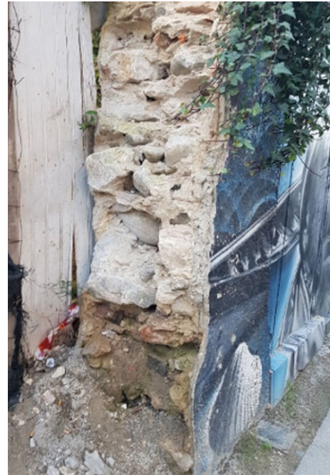
Fig. 2. Section of formed masonry with lime mortar, width of wall 0.52 m (© Alice Tavares).
