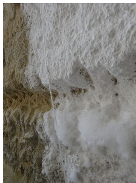
Fig. 13. Detail of salt efflorescences in test area (image height match – 50 cm) of adobe wall after seven days lime water painting (© Alice Tavares).
