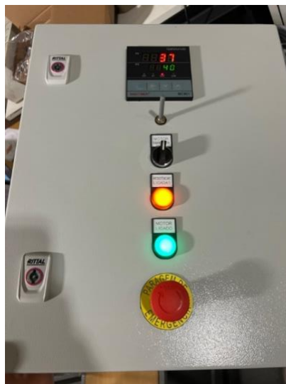
Figure 54 Visible part of the electric panel (Extrusion).
