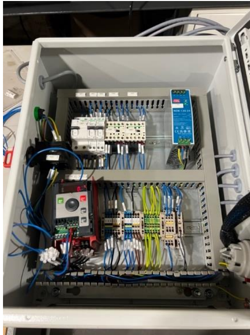
Figure 53 Inside of electrical panel (Extrusion).
