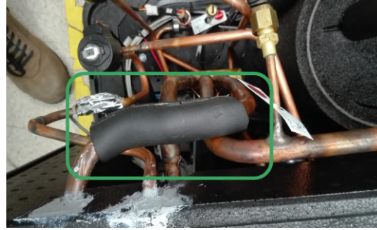
(b) Addition of foam around the gas line inside the compressor module.
