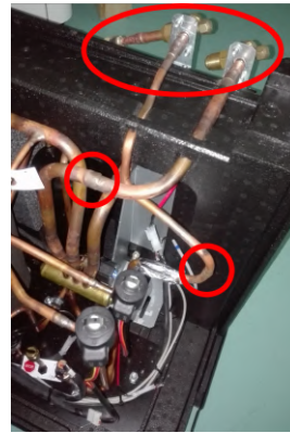
(b) CM - refrigerant circuit re-worked.
