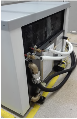
(a) Compressor module - flexible hoses.
