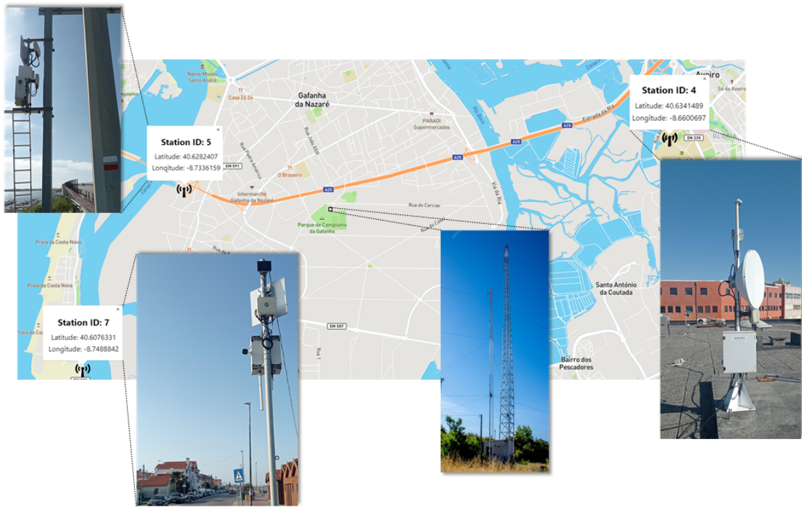
Figure 4.13: RSUs installed with a radio link connection
