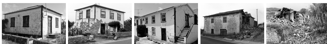
Figure 4.4: Example of observed damage states ds_1 to ds_5 based on the classification proposed by Neves et al. [185], from left to right, which correspond to slight cracking, moderate cracking, extensive cracking, partial collapse and ruin, respectively. Source: Faial database.
