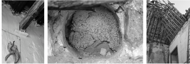
Figure 3.11: Examination of timber joists support on load-bearing walls (left) and the connection between the roof structure and perimetral walls (right), through direct visual inspections and local sampling.
