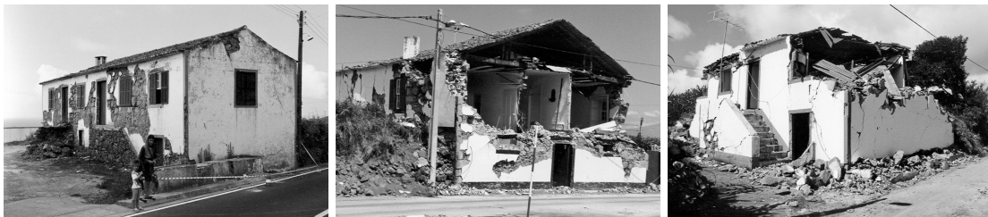
Figure 4.1: Illustration of the damage observed in the sequence of the 1998 Azores earthquake in some of the most affected parishes of Faial Island: Castelo Branco, Flamengos and Pedro Miguel (respectively from left to right). Source: Faial database.
