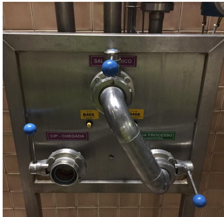
Figure 34 U pipe and adjacent valves showing the connection between the process water pipe to the wort production area and the close connection from CIP products
