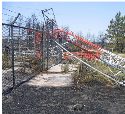
Figure 4.5: Destroyed communications tower, caused by a wildfire.
