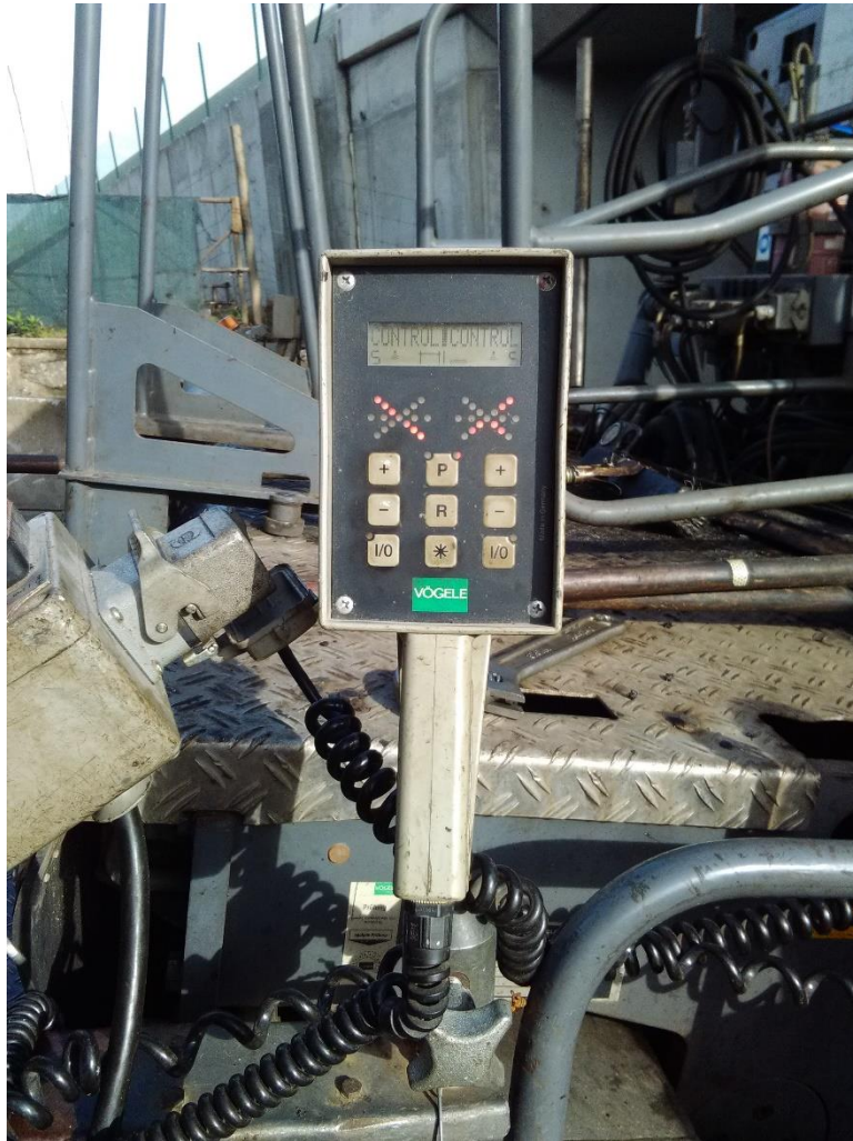
Figure 4.8 – Paver's Electronic Control System
