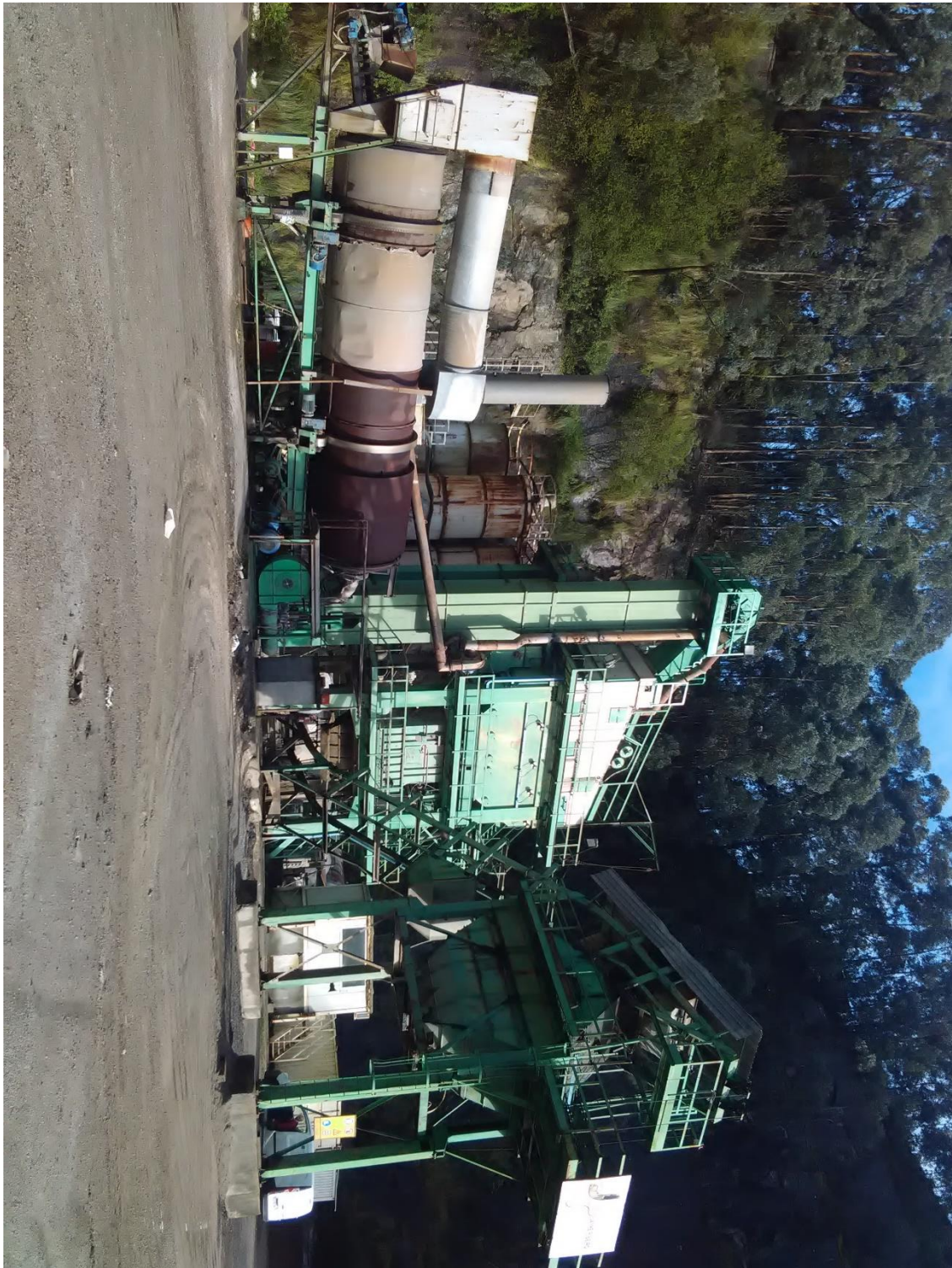
Figure 4.2 – Mixing Plant Used
