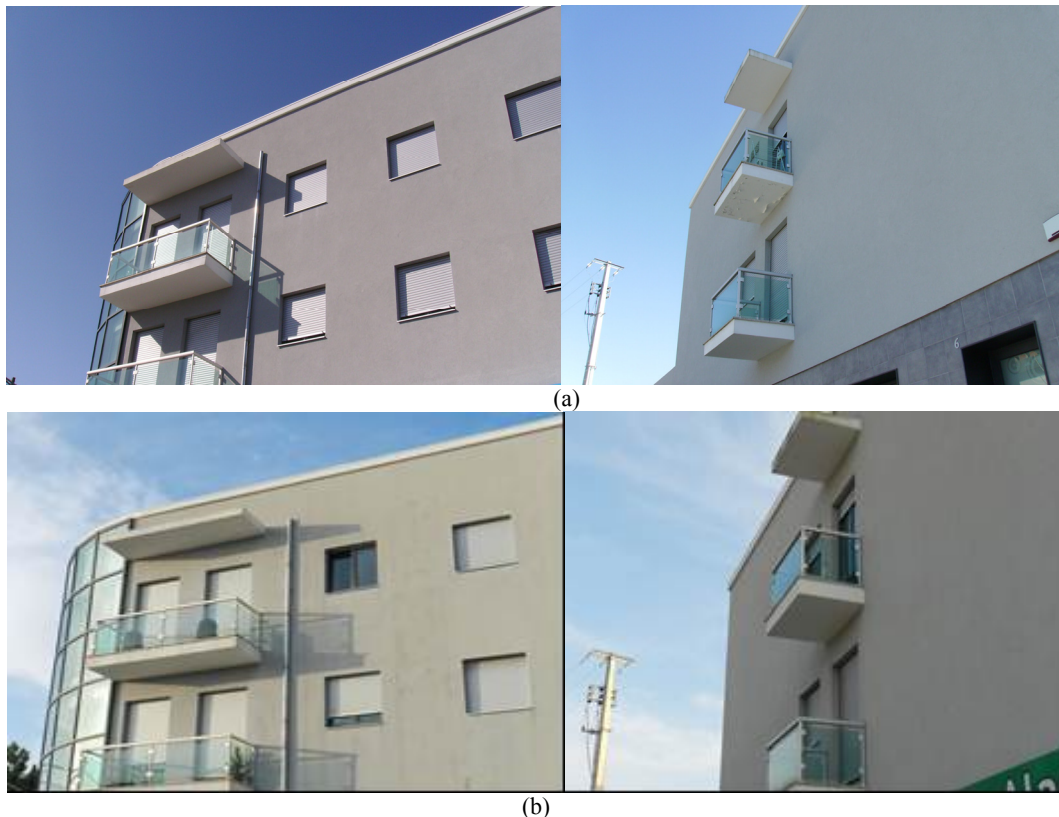
Fig. 4 Visual inspection of in situ evaluation of ETICS: (a) beginning and after 4 years; (b) 6 years exposure conditions (left: south orientation; right: north orientation).
