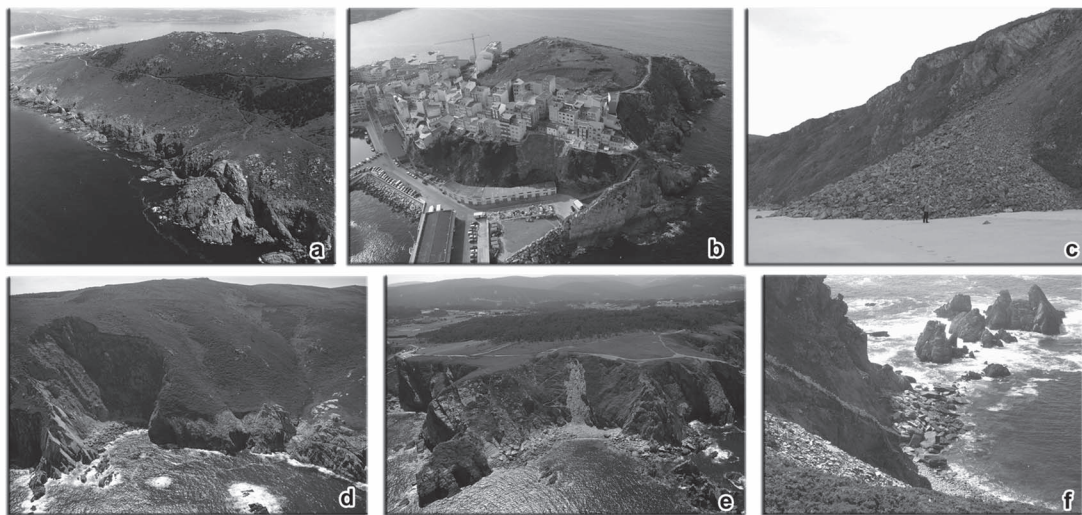
Figure 6. Stability level along the rocky coast and some examples of mass movement ((a) Fisterra; (b) Malpica; (c) Ferrol; (d) Cabo Ortegal; (e) Ortigueira, general view; (f) Ortigueira, detail). Black
