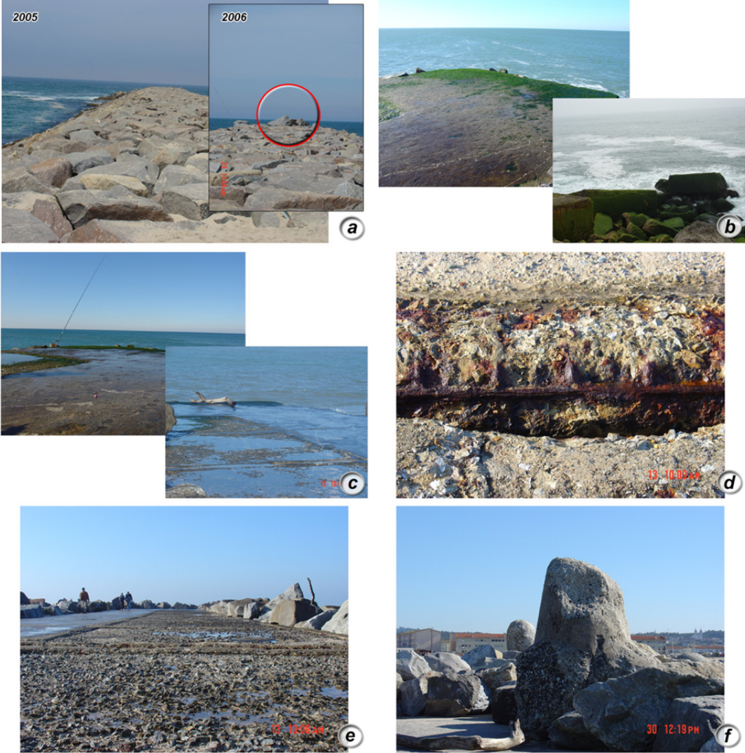
Figure 48. Visual observation of Espinho field groynes (NW Portugal): (a) displaced stones and differences along the armour layers component; (b) and (c) potential problems and breakage and cracking; (d) and (e) corrosion of the concrete material or symptoms of deterioration; (f) concrete material broken armour units.
