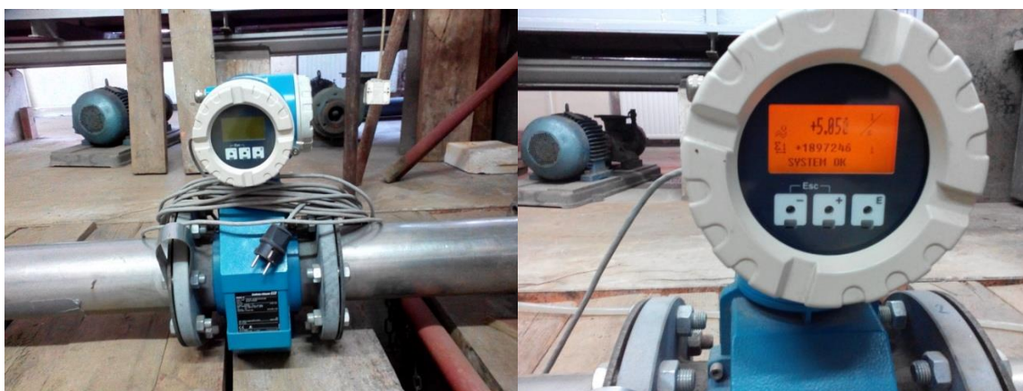
Figure 60. Electromagnetic flowmeter utilized to measure the flow discharge.
