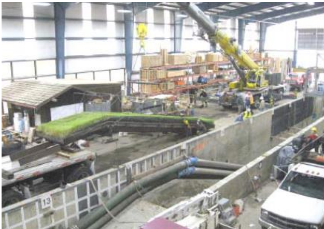
Figure 38. Metal tray with vegetated HPTRM system being installed on the dike inside the flume (Amini and Li, 2012).
