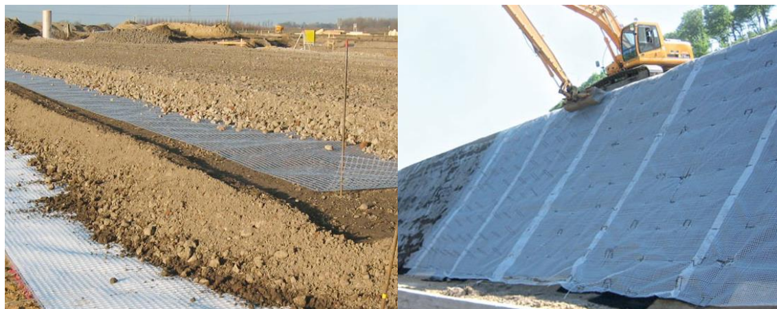
Figure 59. Application of a composite product of a geogrid and geotextile (Combigrig ® ) for soil reinforcement (on the left picture) and application of a geogrid layer only with U-shaped fasteners over a steep slope (on the right picture) (figure extracted from www.naue.com , 2013).
