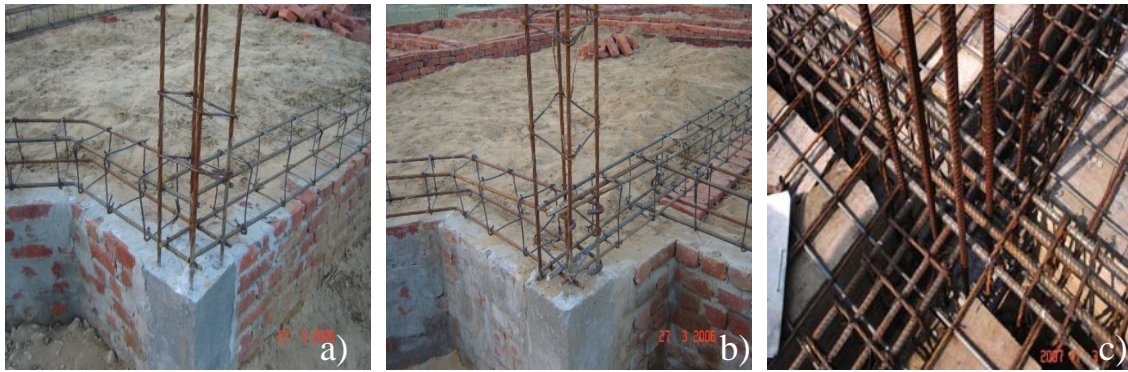
Fig. 1 a) No anchorage of beam bars in column b) Beam reinforcement hooking into column reinforcement c) No stirrups in beam-column joint
