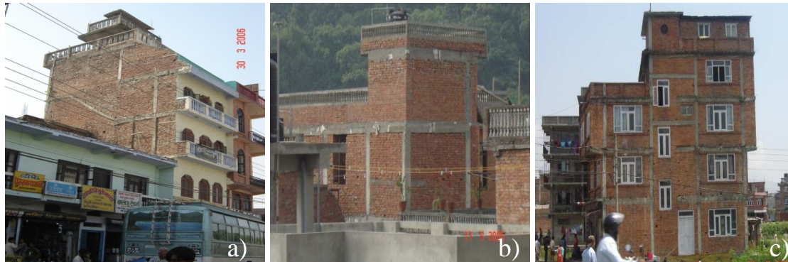
Fig. 4 a) Column starting from fifth storey b) Missing column in top storey c) Missing beam
