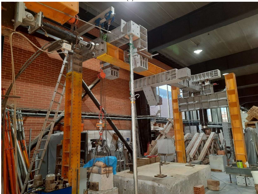
Figure 2. Cyclic shear test system for full-scale walls: (a) illustrating out-of-plane tests and (b) prepared for in-plane tests.
