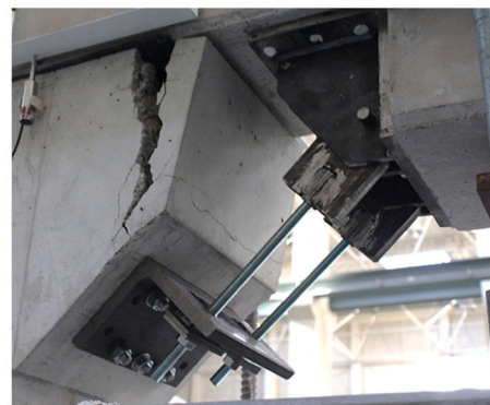
b) Corbel damages
