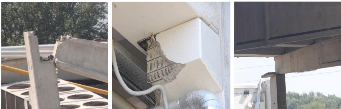
Fig. 1. Examples of beam-to-column connection failures in precast industrial buildings.
